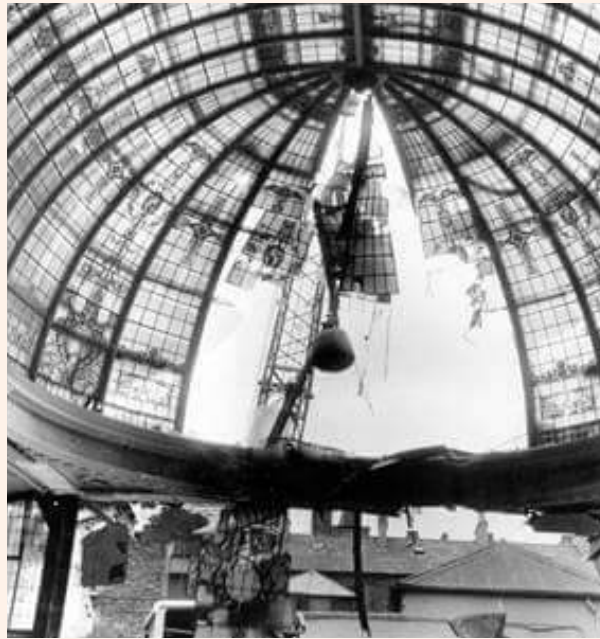
The old Northern Bank branch on Donegall Square was demolished to make room for the new one.
